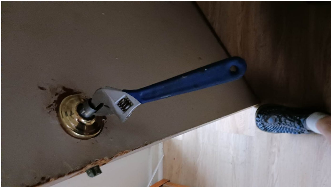
Figure 2: Door missing its knob, with an adjustable wrench applied to the remaining brass hardware. Wear and damage are visible along the door edge.
