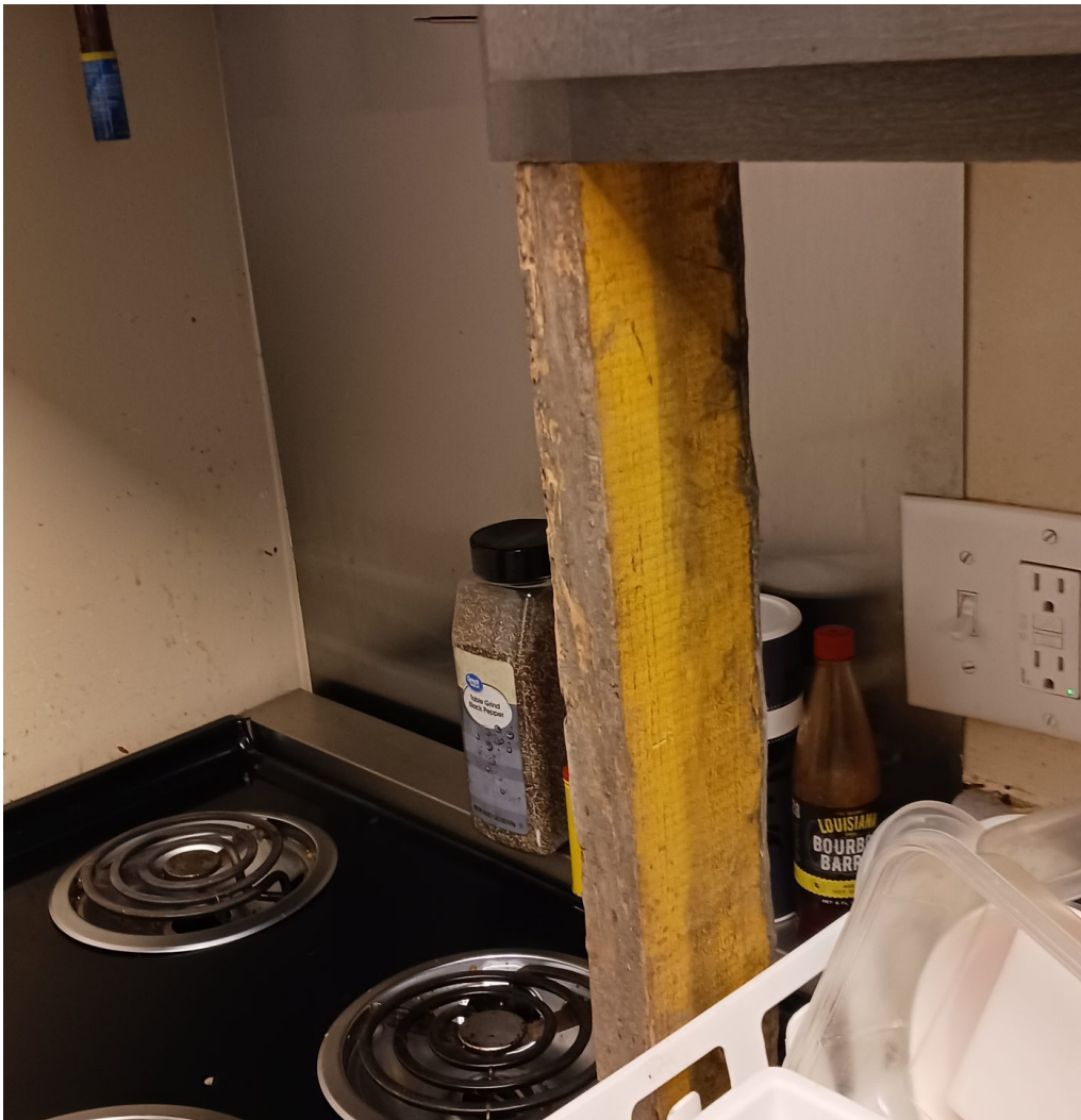
Figure 3: Rough wooden plank (with yellow marking) propping up an upper cabinet/shelf immediately above an electric stove at Central Park Tower. The support is in the cooking area.
