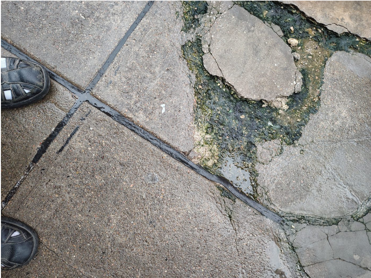
Figure 4: Deteriorated exterior sidewalk at Central Park Tower showing missing concrete, cracks, standing water, and surface growth. The condition creates trip and accessibility hazards.
