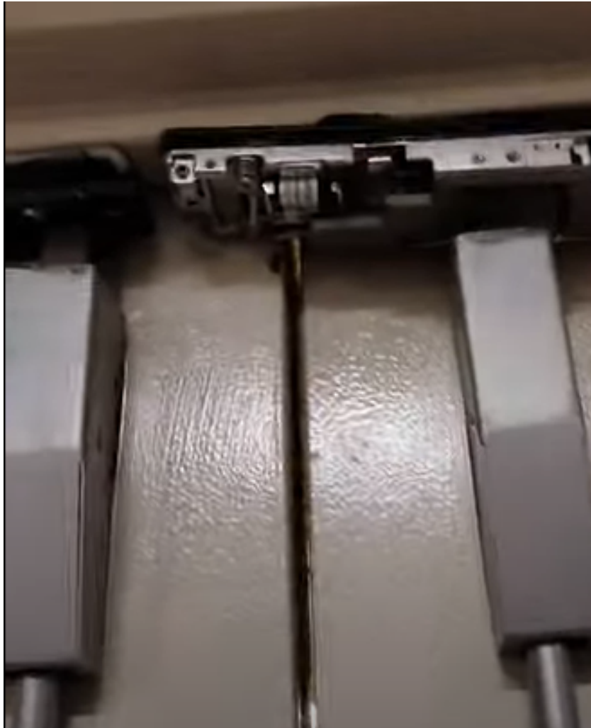
Figure 2: Close-up of the lock edge. Internal hardware is exposed. The latch/bolt assembly is not a complete, working commercial lockset. The door cannot be secured with a key or hasp in the condition shown.
