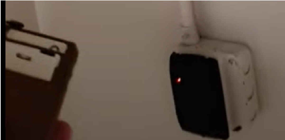
Figure 3: Wall-mounted card or fob reader with a red lamp. A credential is held up to the device. The red light is consistent with denied or inactive access, not a working resident key system for the room.
