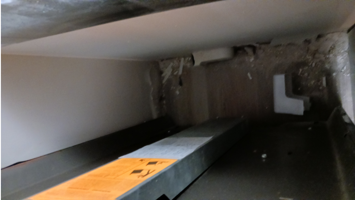
Figure 12: Kitchen opening with debris on the floor. No range or cooktop is installed. No power cord is present to plug in. This photograph answers the claim that a stove was merely “unplugged.”
