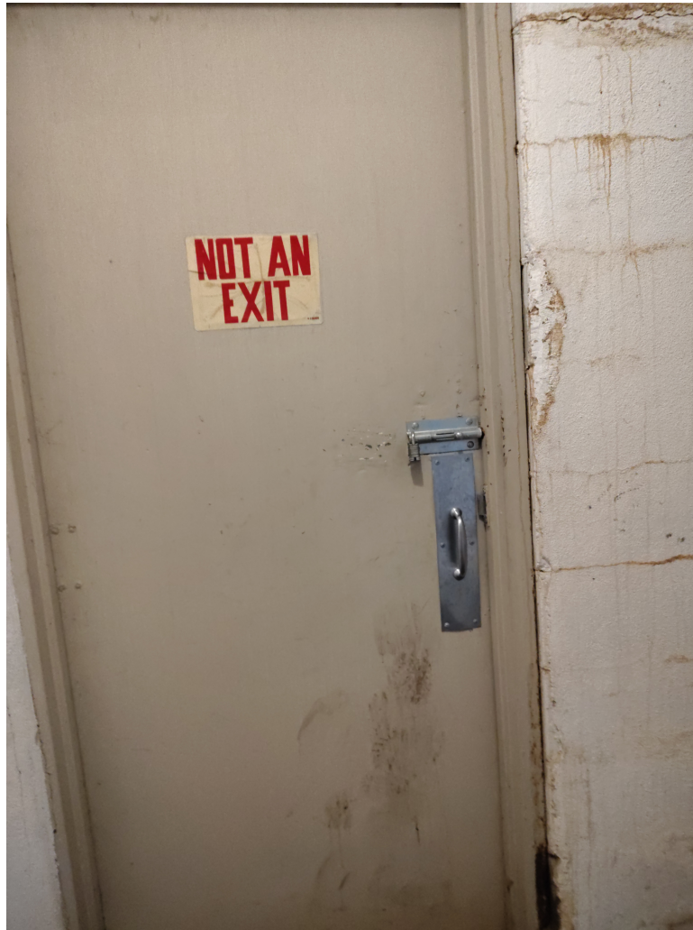
Figure 2: Door with a paper sign reading “NOT AN EXIT,” and a hasp mounted on the occupied side. Photograph, October 5, 2026. The file labeled rooftopdoorblocked.jpg is the same door.
