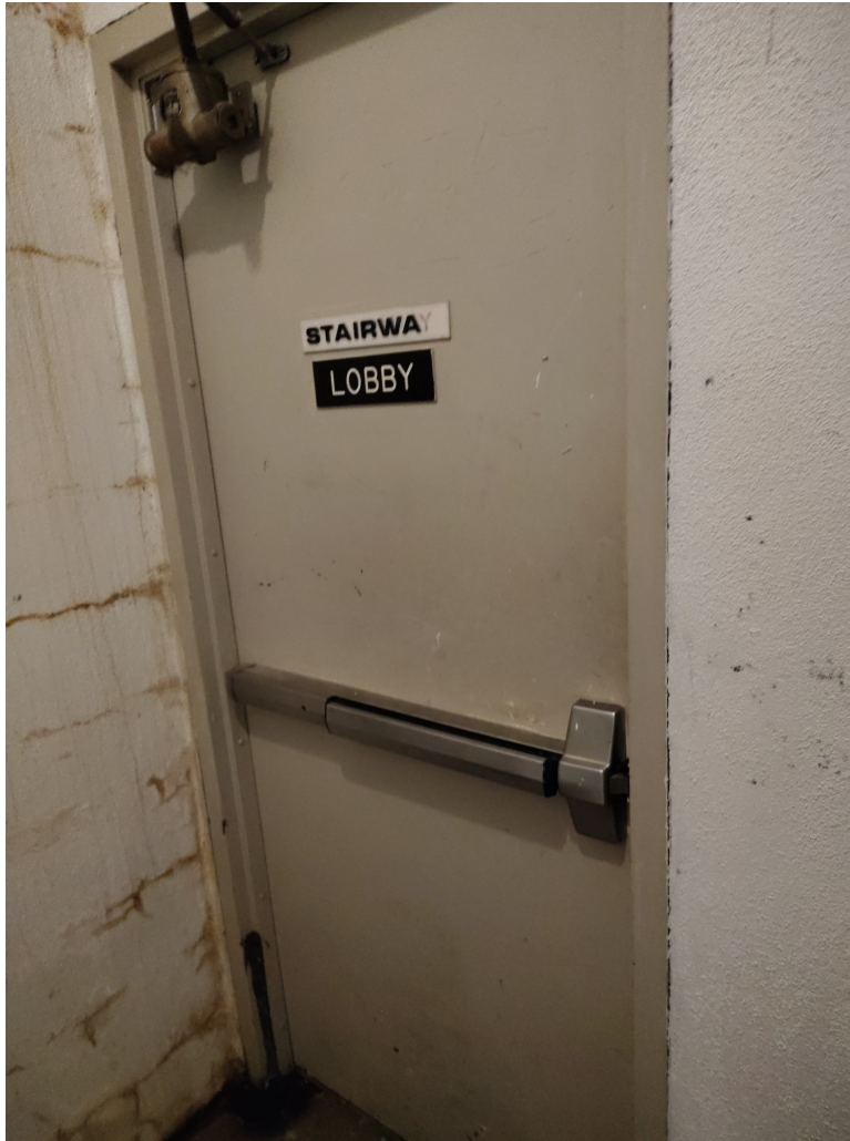
Figure 3: Door signed “STAIRWAY” and “LOBBY,” with a panic bar. A closer or alarm device is at the top of the frame. Photograph, October 5, 2026, Central Park Tower.
