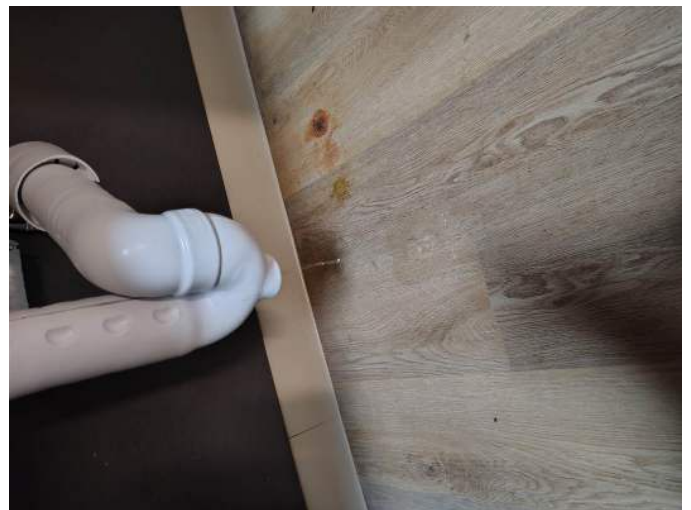
Community room. Bucket under a sink. Cabinet stained.
