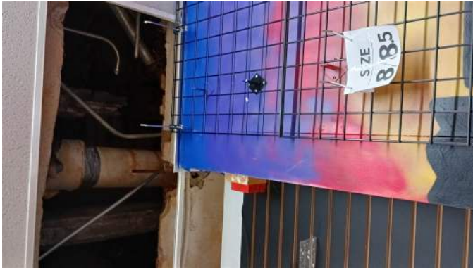
Commercial space at the tower, signed shoe store. Standing water across the floor.
