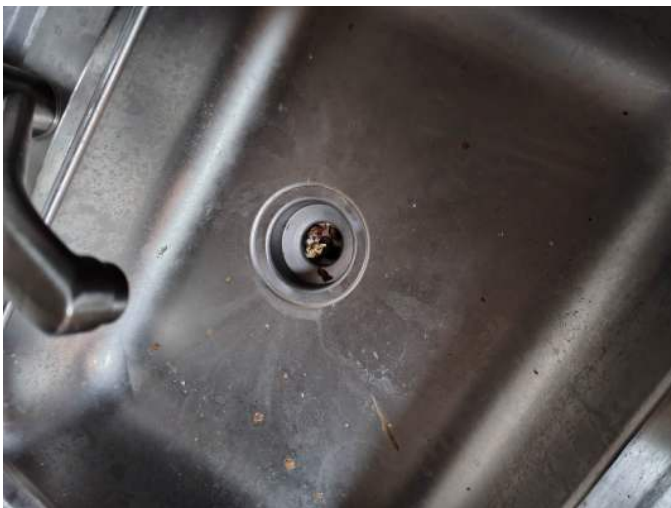
Community-room sink. Basin and wall stained. Faucet in place.
