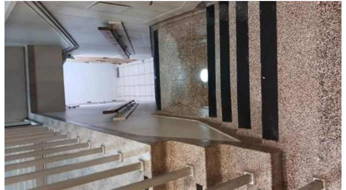
Lobby. Water on the floor at the basement opening.
