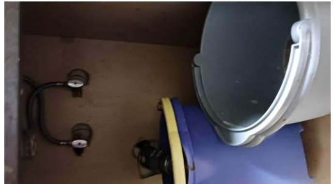
Bathroom. Sink basin stained. Supply line and drain trap exposed.
