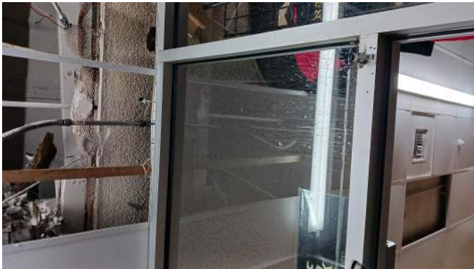
Same space. Water against the interior door.
