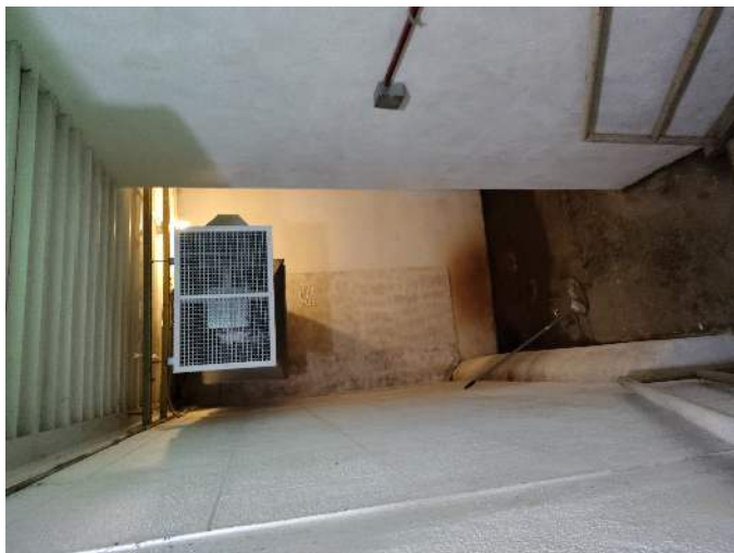
Stair landing. Floor wet. Unit heater overhead. Mop on the floor. No padlock in this frame.
