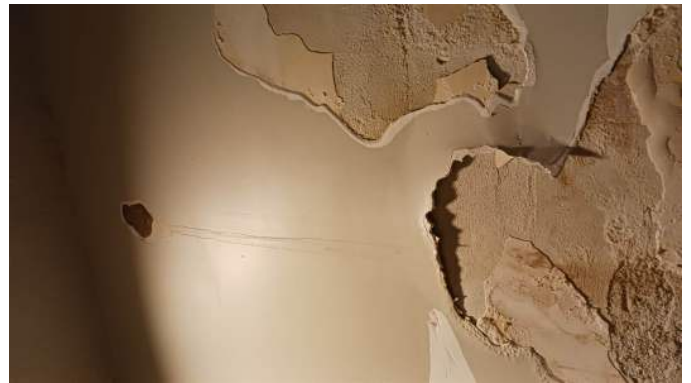
Wall beside that landing. Paint peeled to the block. Stain at the base.
