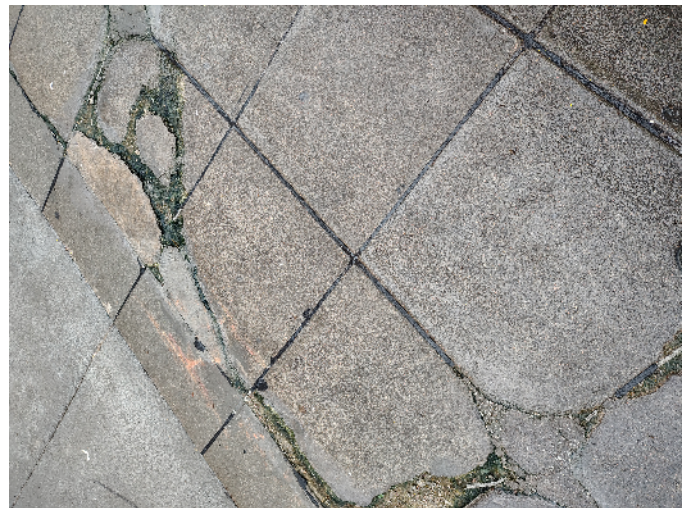
Sidewalk, second frame. Faulted joints and missing panel pieces.
