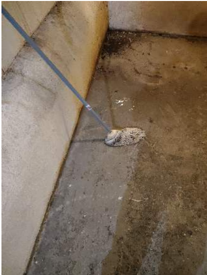
First-floor landing corner. Floor wet. Mop in the water. Walls stained.
