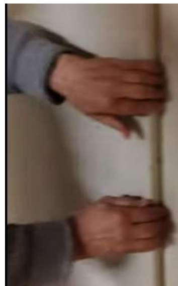
Door edge held open by hand. Gap along the stop.
