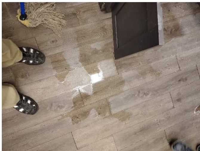
Laundry room. Standing water on the floor. Mop at the edge.
