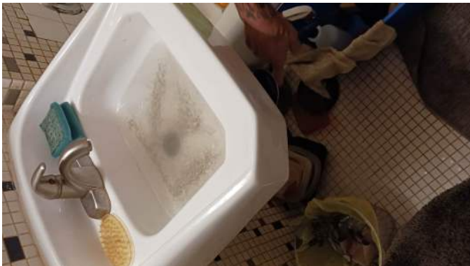
Bathroom. No lavatory. Supply lines and open drain in the wall.
