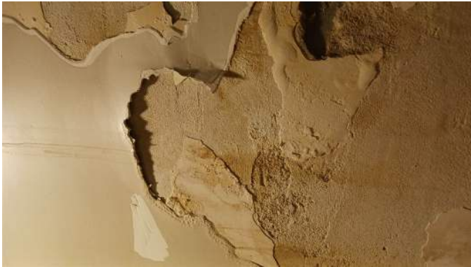
Common-area wall. Paint peeled in sheets. Dark stain on the lower wall.
