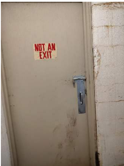
Door signed "NOT AN EXIT." Hasp on the occupied side.
