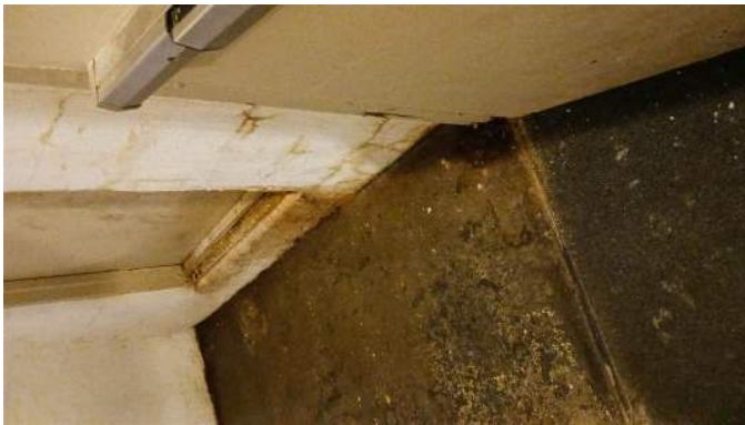
First-floor landing. Door signed "NOT AN EXIT," hasp on the occupied side. File name identifies the roof exit.
