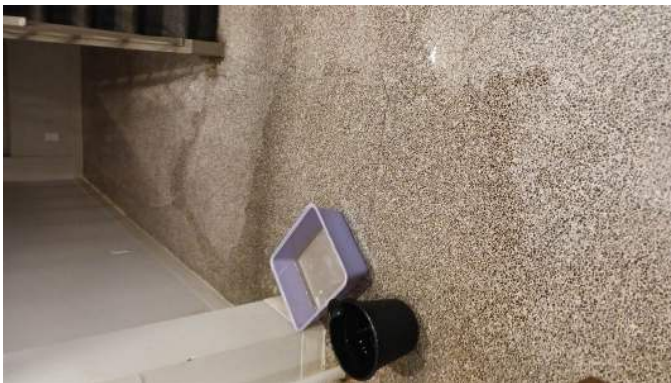
Lobby. Buckets and a trash bin set under leaks. Floor stained.
