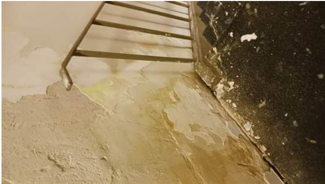
First-floor stairwell. Stairs and landing wet. Caution tape across the flight.
