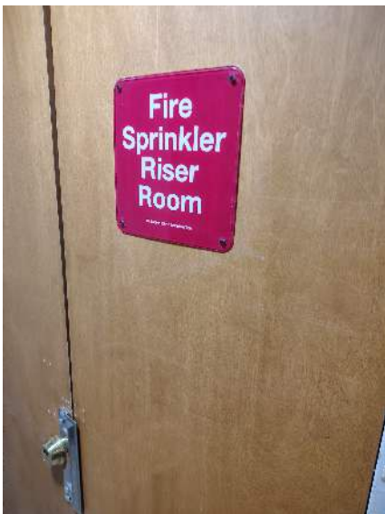
Door signed Fire Sprinkler Riser Room, IFC Section 606.1.1. File name identifies this as the room the sidewalk leaks into. The flood is not in this frame.
