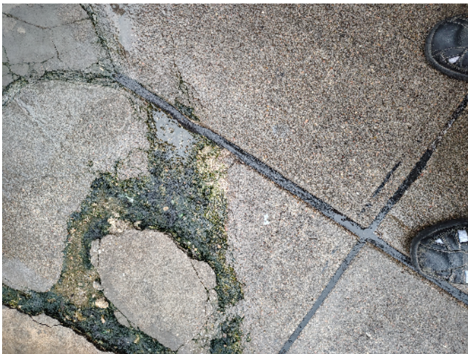
Sidewalk. Open joints, broken panels, standing water, algae in the gaps. October 6, 2026.
