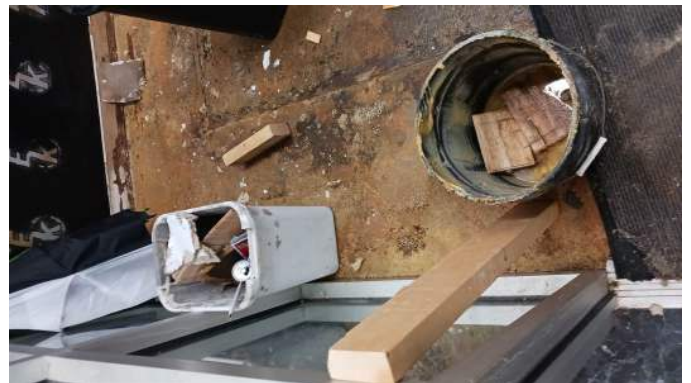
Shoe-store space. Water at the base of the glass.
