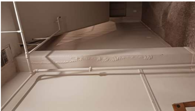
Lobby. Standing water on the floor. Same frame as lobbyfloodedfloor.jpg.
